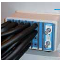
Transits for generator.
