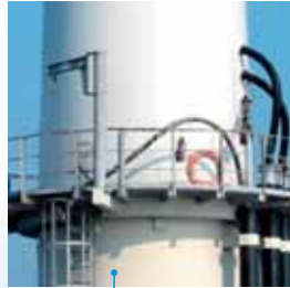
Transits for submarine cable in monopile.
