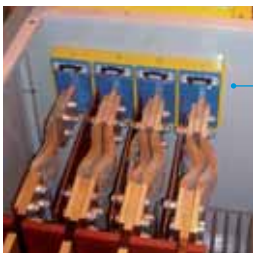
Bus bar transits for transformer room.
