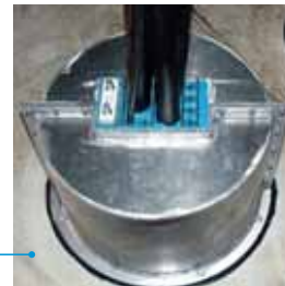
Transits for submarine cable in foundation.
