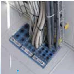
Transits between fire zones in offshore substations.
